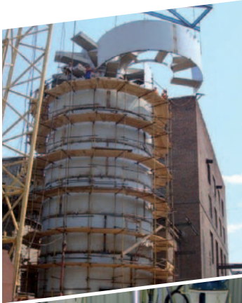
Tower Diffuser Assembly
